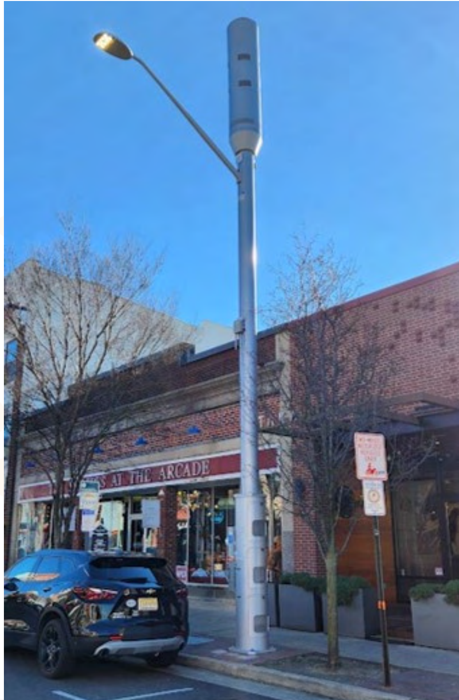
Mid capacity, multi-tenant telecom with roadway lighting brings small cell deployments to the high traffic areas that demand wireless service the most.
